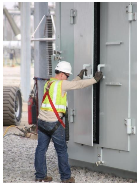
Figure 2 The system allows for easy access to key components during operation of the transformer.
