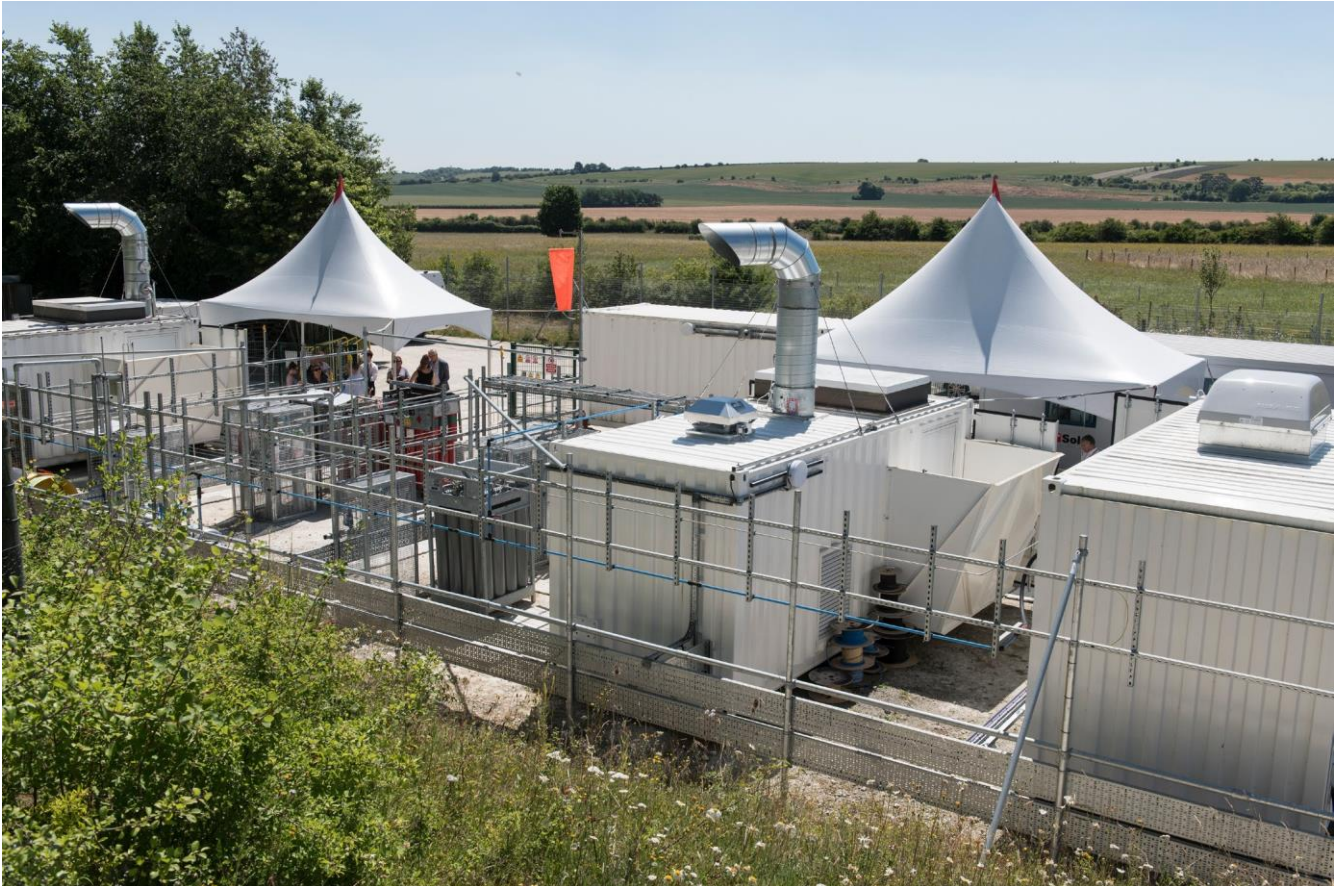
1 Siemens Energy e-Ammonia demonstrator at Rutherford Appleton Laboratory in Oxfordshire, UK. Picture courtesy of the Science and Technology Facilities Council, UK.
