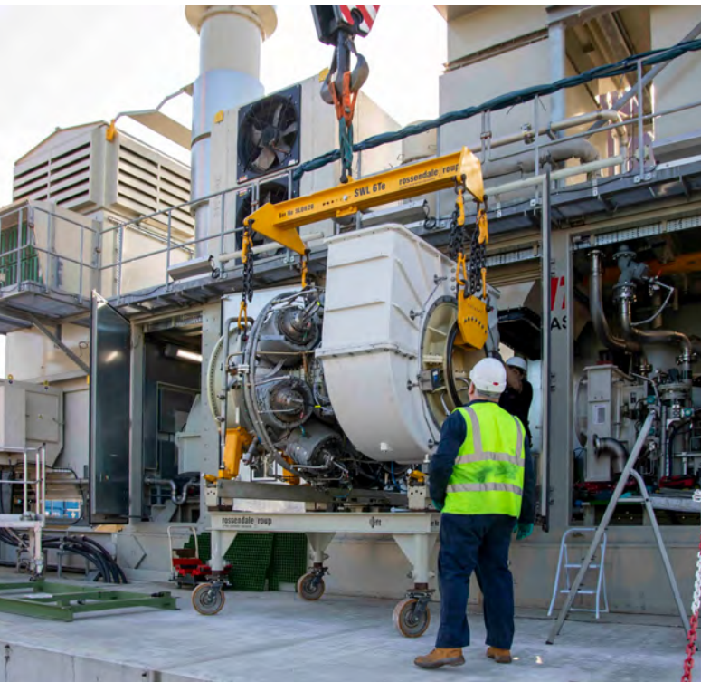
Figure 5: Installation of SGT-400 core engine at the HYFLEX-POWER demonstration plant in Saillat-sur-Vienne in France
