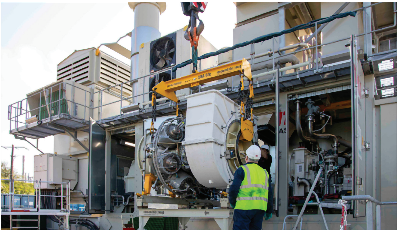
Figure 3. SGT-400 gas turbine at Smurfit-Kappa paper plant. Gas turbine combustion system was modified to burn hydrogen/natural gas blends up to 100% hydrogen content.
