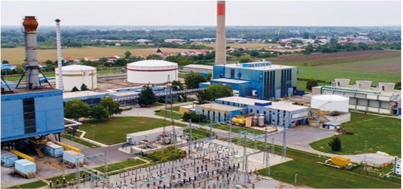
TE-TO Osijek, Thermal Power Plant
