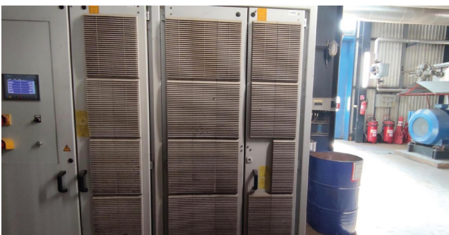
TE-TO Osijek, Variable Speed Drive
