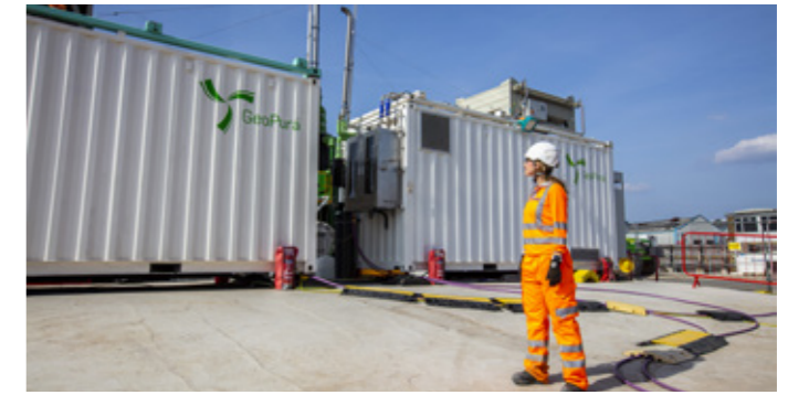
GeoPura hydrogen power units are providing hydrogen-fueled clean energy.
