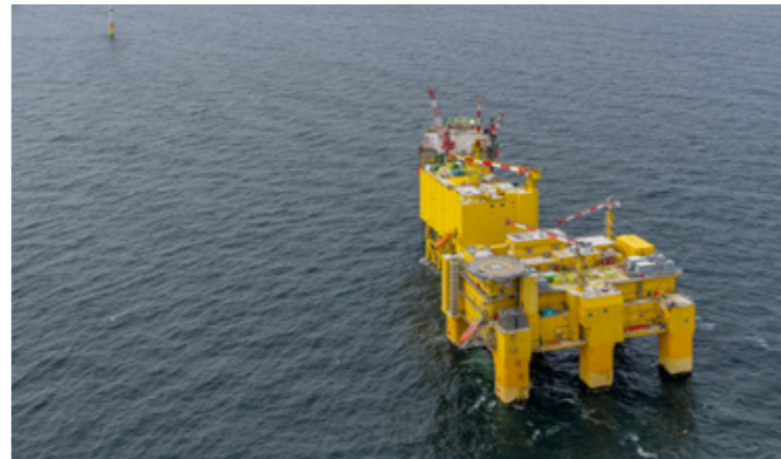
Successful installation in the North Sea: Providing more than 1 million households with green wind power.
