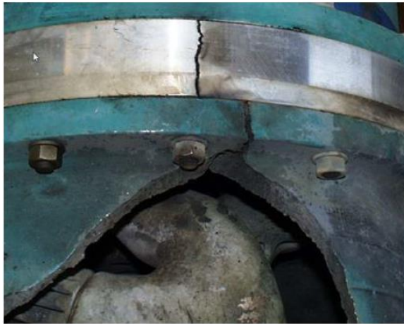
Figure 2: Fragmentation at a GIS enclosure.
