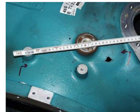
Figure 2: Hole and tear in a GIS enclosure.
