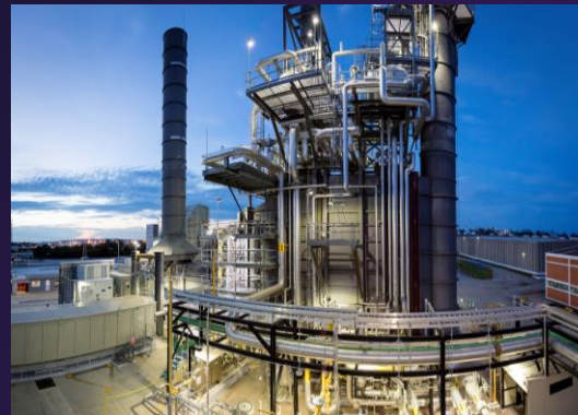
Modern Gas Power Plant with combined heat and power technology / H 2 co-firing
