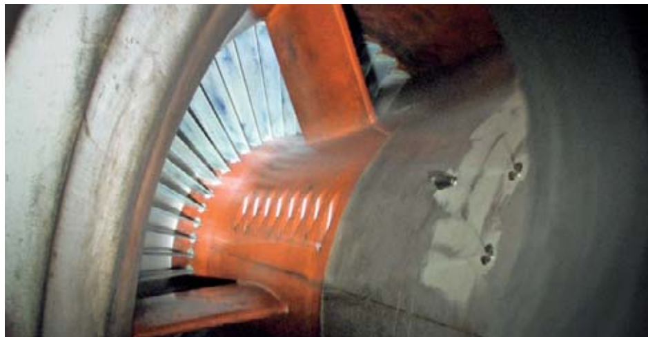
Air intake inner cone with nozzles – on-line washing
