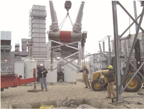
Figure 2 Turnkey breaker replacement with Siemens Energy SPS2
