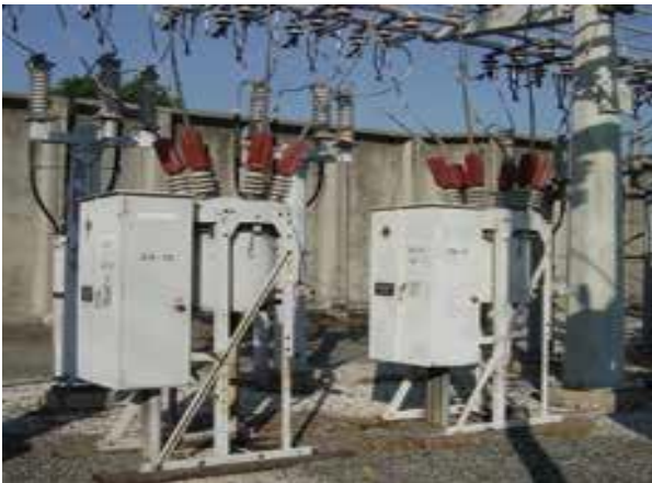
Figure 3 Siemens-Allis 30kV SDO circuit breaker
