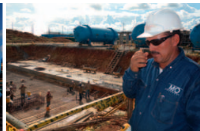
Siemens Engineer Félix Suárez in front of a flotation cell for the new water purification complex that the company is helping to build at Acacias (left). Work is proceeding on the enormous underground tank for the Ecopetrol facility (right).
