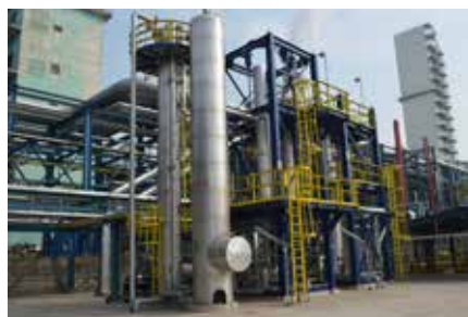
Zimpro® WAO unit at Jiujiang plant
