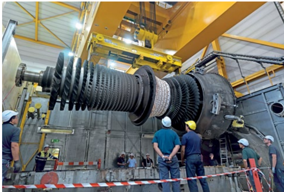
Comprehensive on-site field service
