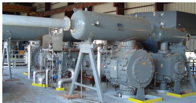
A typical Dresser-Rand HHE-VL reciprocating compressor installation utilizing an engine-type synchronous motor similar to the configuration of the three units that will be installed at a steam methane reformer in Texas.
