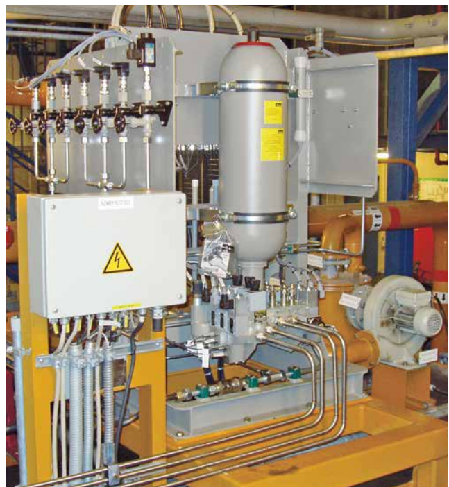
Hydraulic Clearance Optimization pump skid
