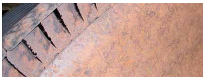
Heavy corrosion of rotor
