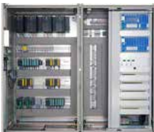
(TURLOOP) Turbine control cubicle
