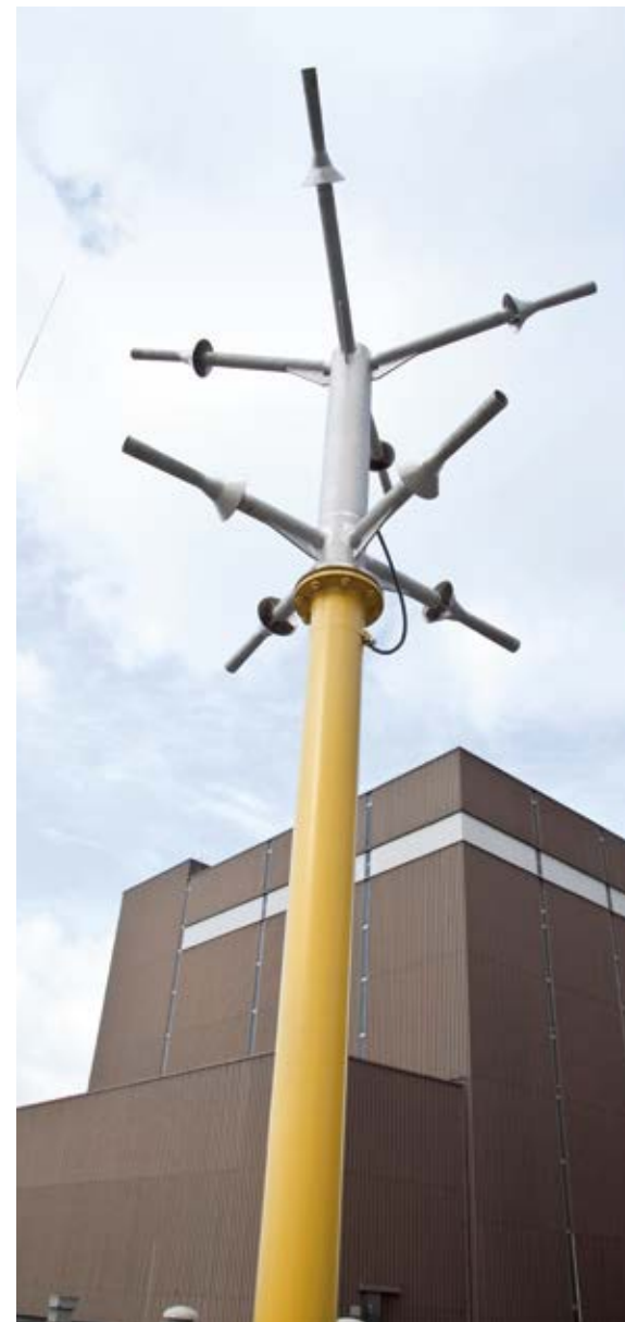
Installed vent star with equipotential bonding
