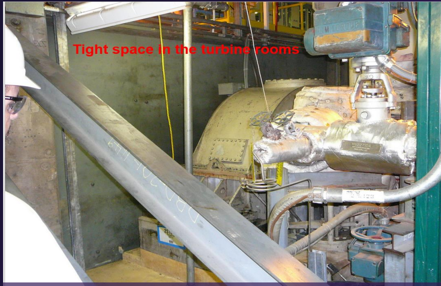
Initial study where the engineer is working to identify the ideal SST-DR turbine type that has 10% increased output power as per customer requirements but at the same time fit in to the existing tight spaced turbine rooms
