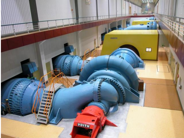
Power Plant Wehr, generator (4 x 300 MVA)
